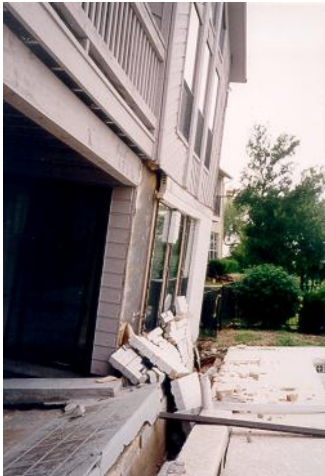
Pool deck down dropped and pulled away from house during landslide.
