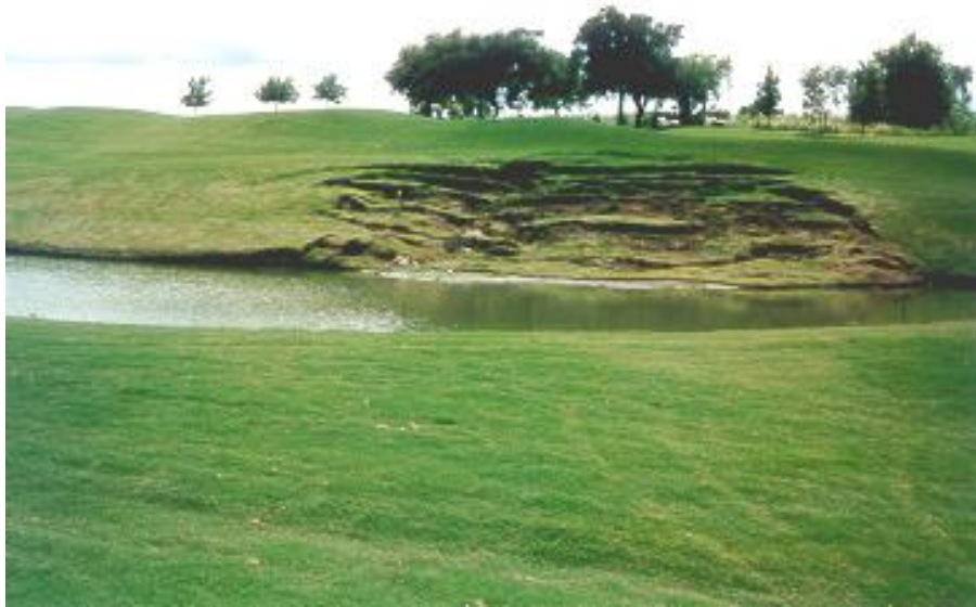
Failed slope at golf course in Plano.
