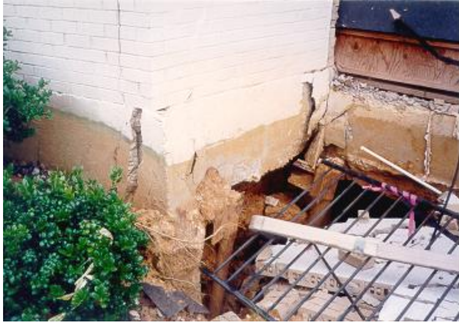
Broken foundation along landslide scarp.
