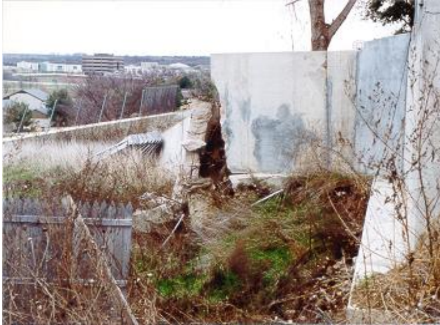
View of broken retaining wall along failure scarp of landslide, Benbrook.
