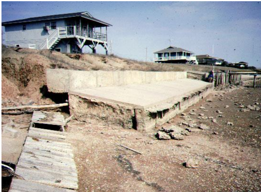
Damage to property due to coastal erosion of clay-rich sediment in Texas back bays can be as bad as damage to structures exposed on the open coast.
