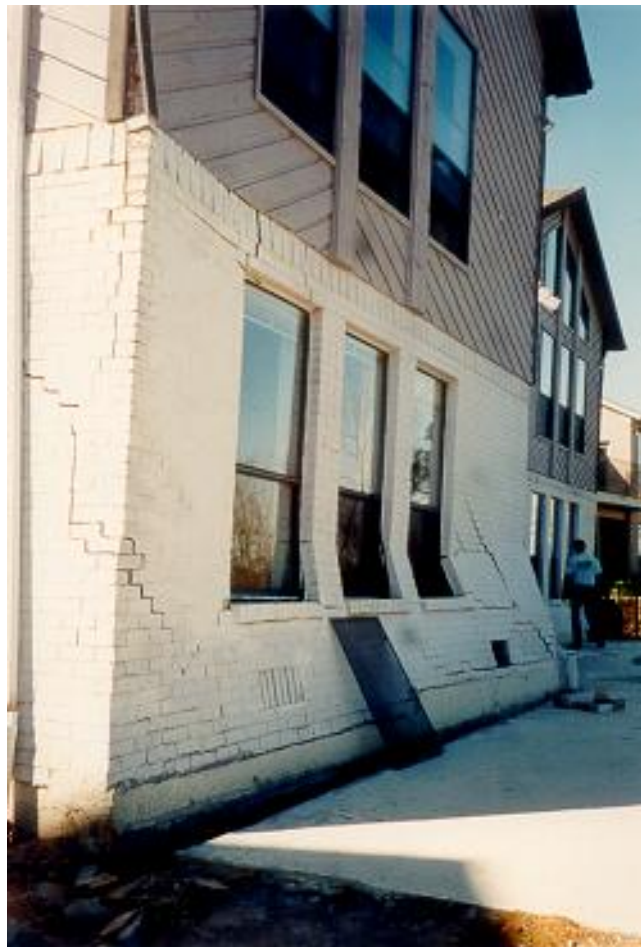
Side of house pulled away at foundation level resulting from movement of landslide.
