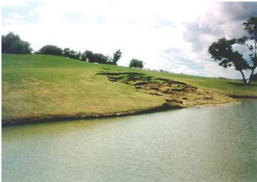
Failed slope at golf course in Plano.
