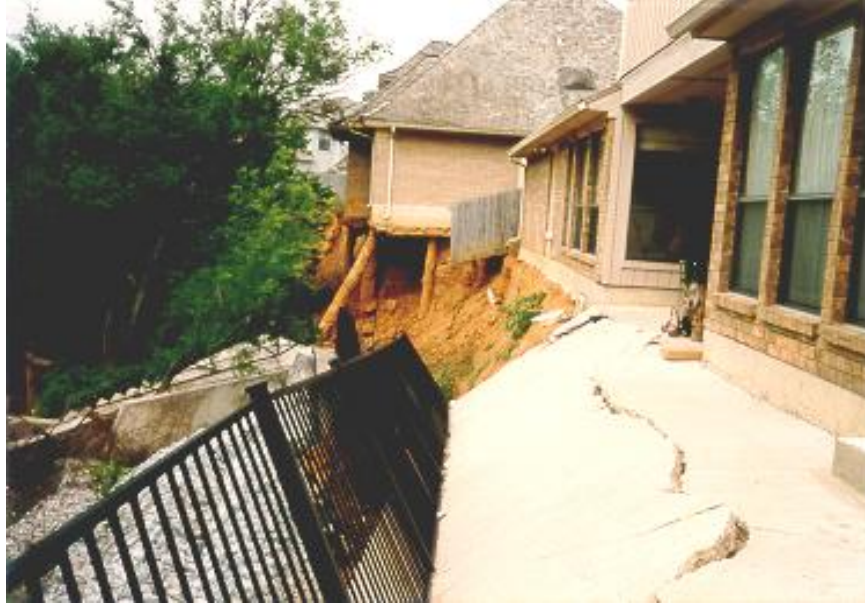
Additional view of damage to home from erosion during 1991 flood, Dallas area.
