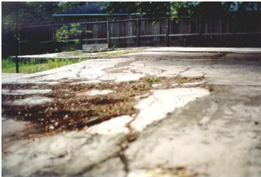
Home foundation built on Long Point Fault at 9131 Olathe in Houston. Note the foundation is broken and has fallen down to the left with movement of the fault. The home had to be demolished.
