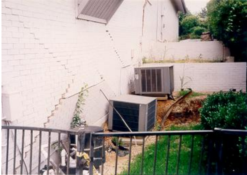
Separated scarp of landslide extending under home in Dallas area showing breaks in wall.
