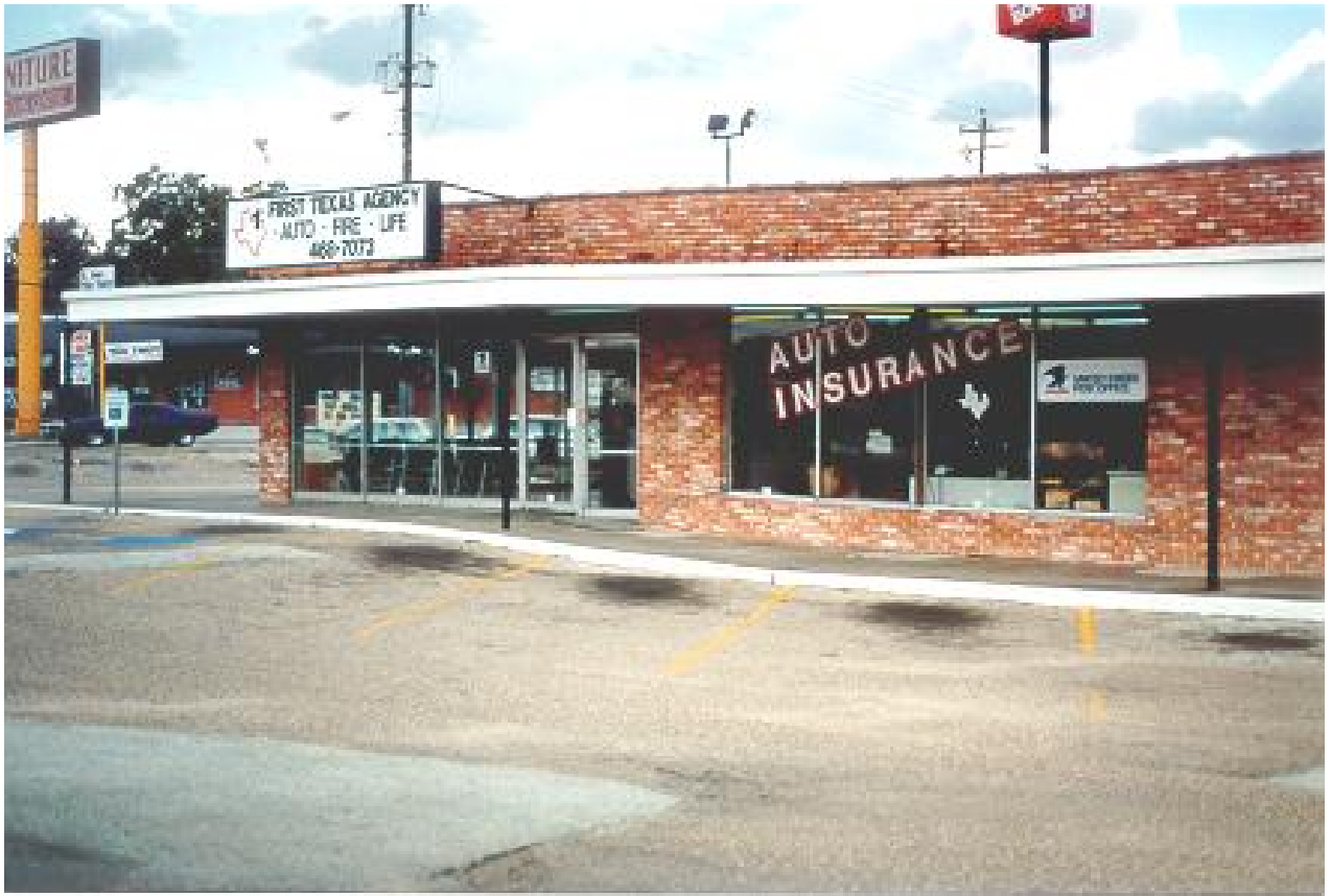
Building constructed on Long Point Fault on the south side of Long Point Road between Peck and Willendahl. Note the drop to the right drop in the driveway. In this picture the fault is downthrown to the right. The building has settled with the fault.
