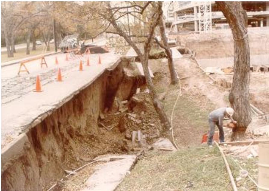
Slide into open excavation on Maple Avenue on November 11, 1984. Note that head scarp has undermined Maple Avenue.
