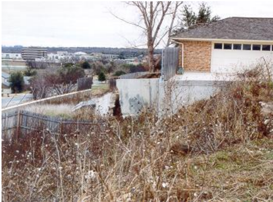
Damage to retaining wall adjacent to home in Benbrook , undermined by a landslide.
