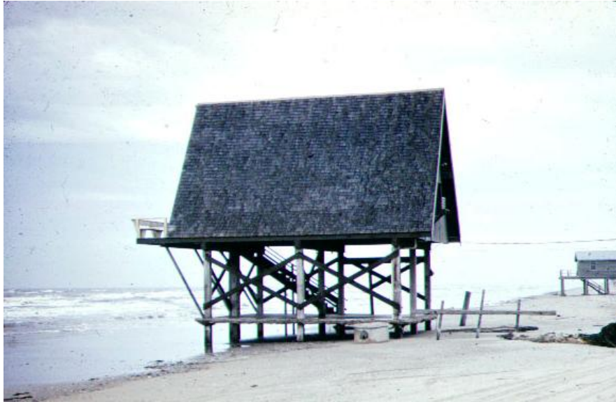
Inadequate assessment of sediment balance led to loss of this coastal home. Note exposed Septic Tank.
