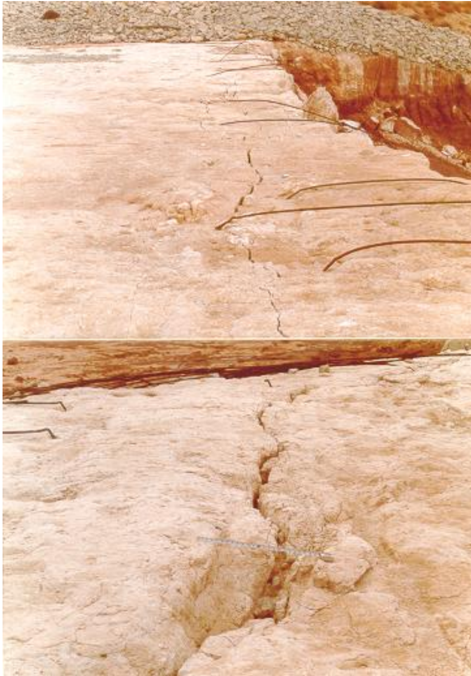
Lake Tanglewood Dam and emergency spillway showing vertical fractures within the rock along the face of spillway.
