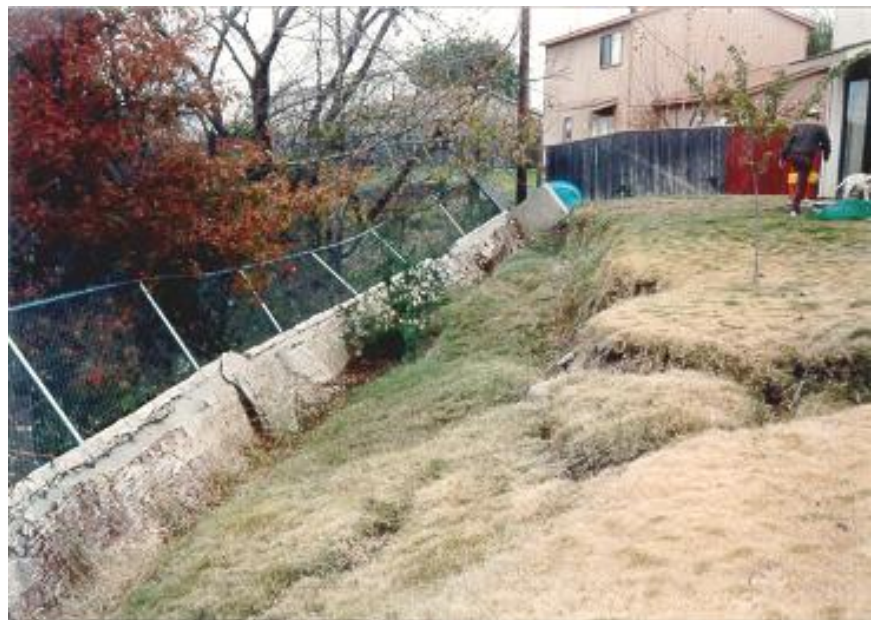
Failed retaining wall behind home resulting from stream erosion at the base of the wall.
