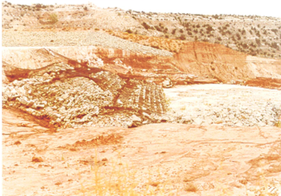
Lake Tanglewood Dam and emergency spillway showing destroyed gabion baskets erosion control improvements.
