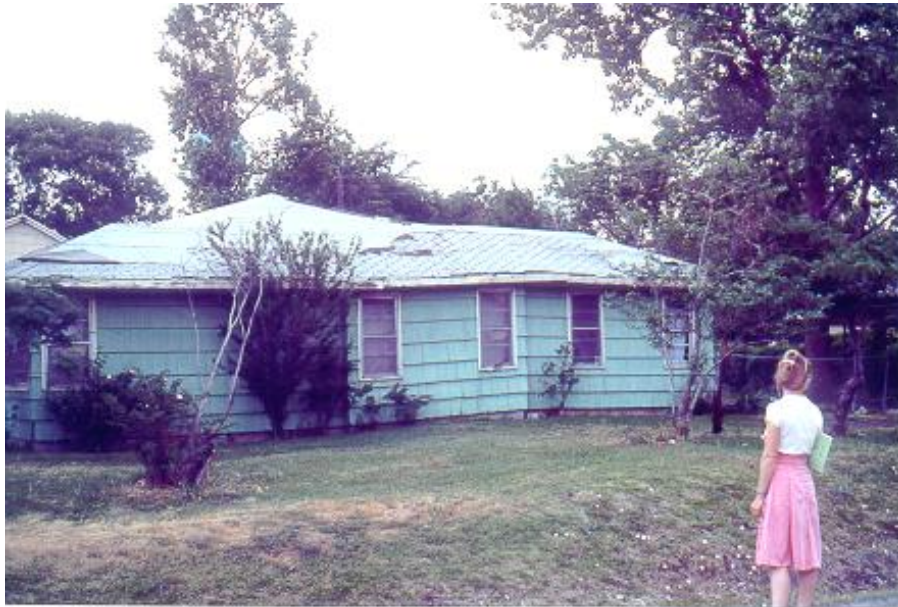
Baytown Texas ó Wooster Fault damaging home at 329 Abbot. Not economically feasible to relevel home. Downthrown fault block is to the left.
