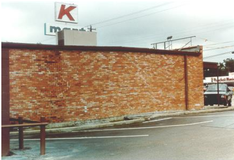
View of structure built on Long Point Fault at the intersection of Long Point and Lynnview in Houston
