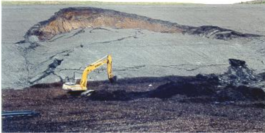
View of the failed western wall of the landfill due to landslide.
