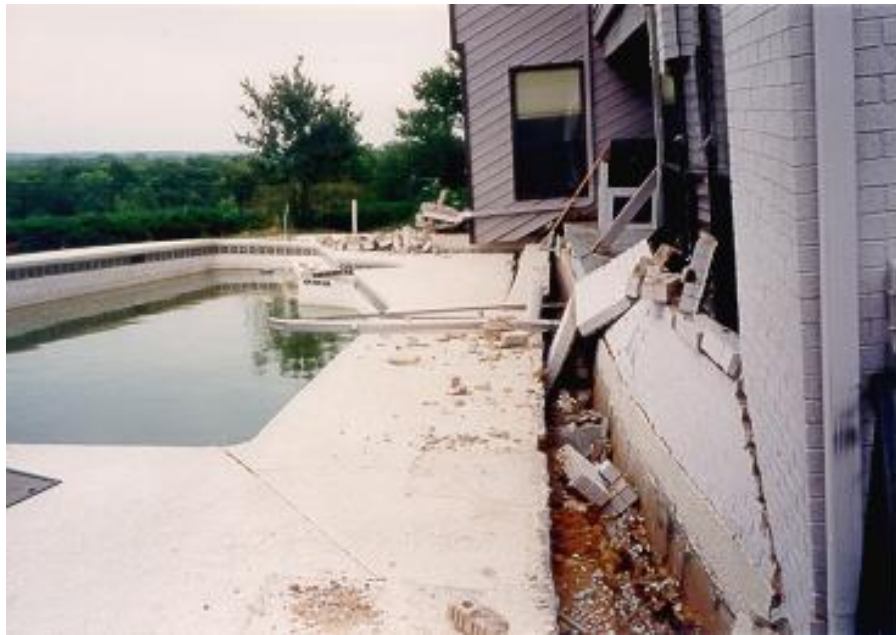
Gap between pool and home resulting from landslide.
