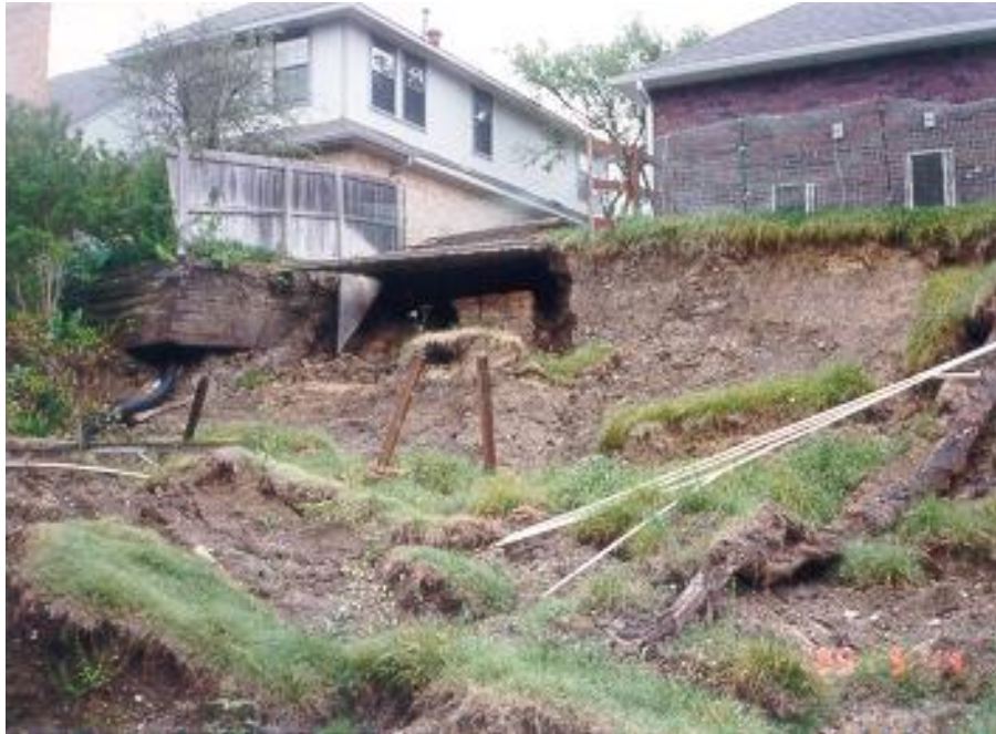
Landslide at home in Carrollton area showing progressive failure of head scarp undermining driveway.
