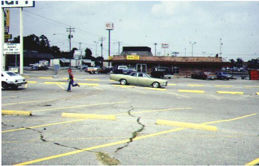
View showing fault traces in pavement associated with subsidence in Houston. Note depressed area to the right.
