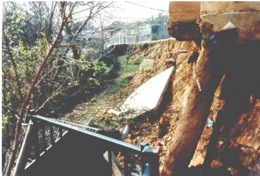
Exposure of pier foundation under home as a result of stream erosion in Dallas area.
