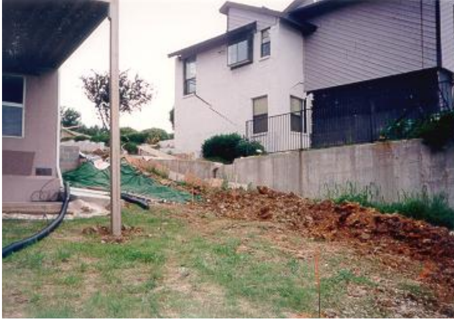
Home damaged by landslide in Dallas area. Note crack in house siding and broken retaining wall.
