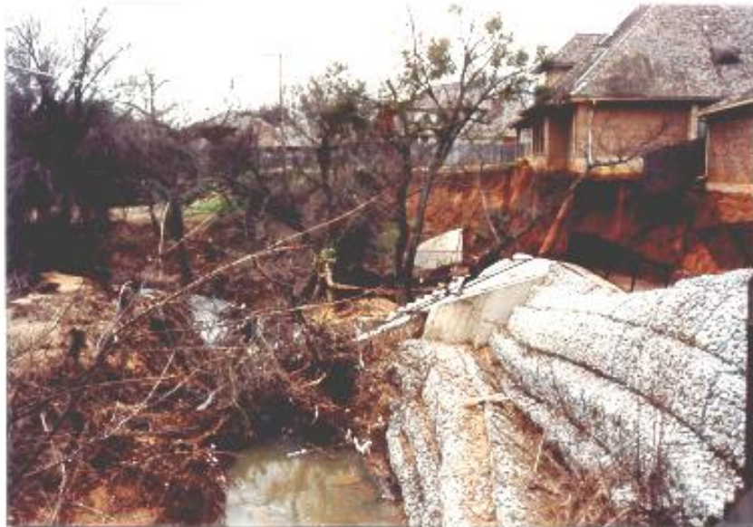
Conditions of erosion control gabion baskets after 1991 flood, Dallas area. Note undermining of home foundations.
