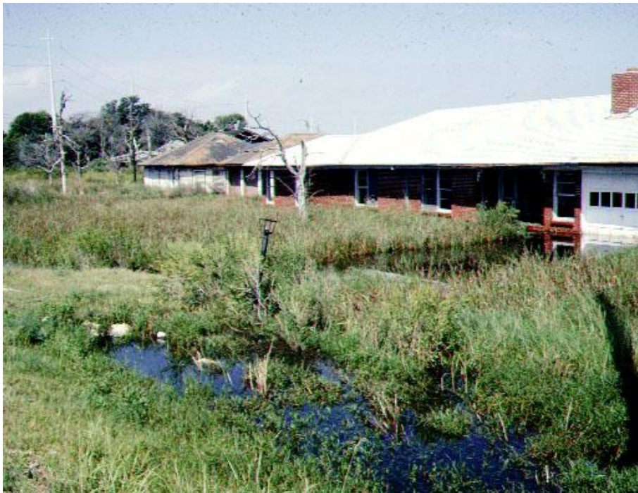
Residence in Brownwood Subdivision ó Baytown. Subsidence of this subdivision area resulted in flooding, and submergence of this home and others in the area. This subdivision was abandoned as a result of the subsidence and subsequent flooding.
