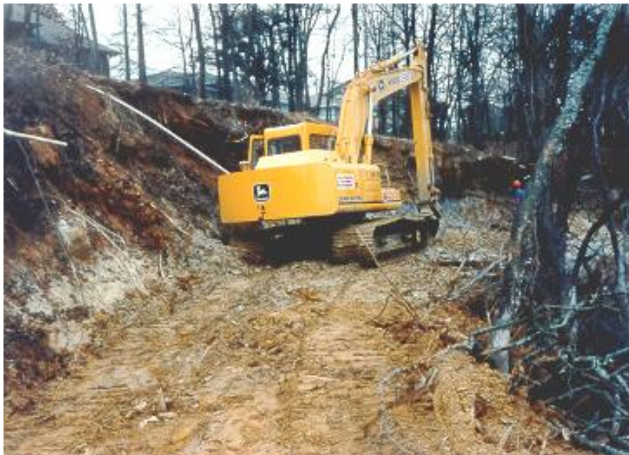
Landslide failure scarp to left of backhoe. Note nearby homes, Grapevine.
