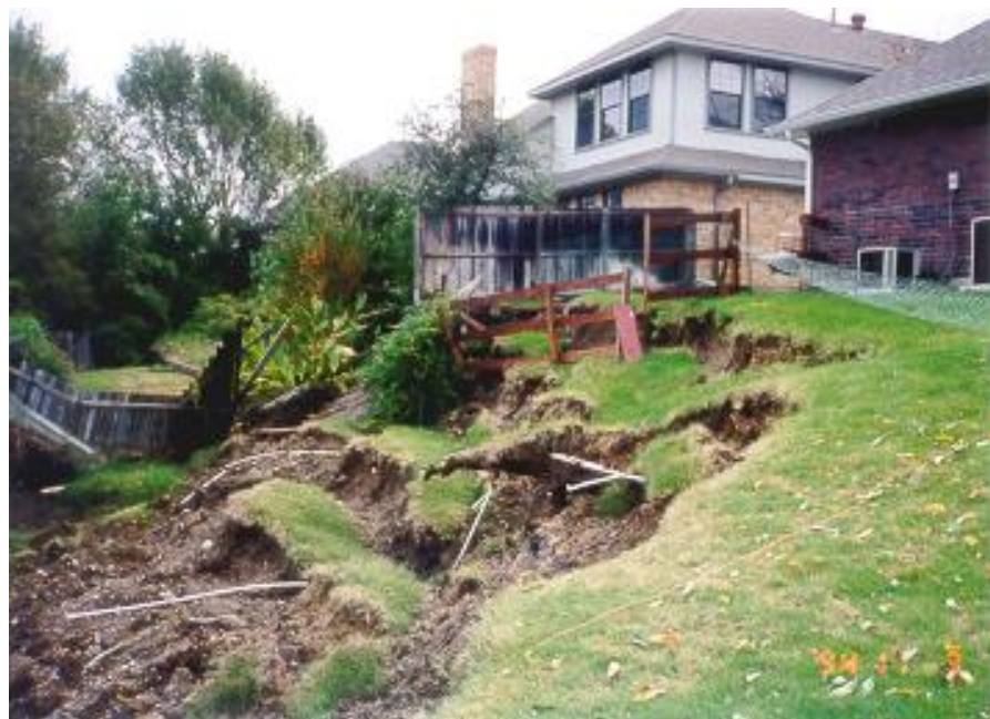
Landslide along creek in Carrollton area showing proximity to home and exposed pipes. The landslide resulted from stream erosion at the toe of the slope.
