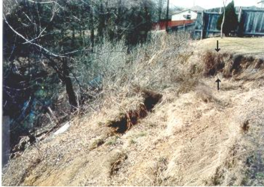
Head scarp of slope failure initiated by stream erosion at the base of the slope along creek.
