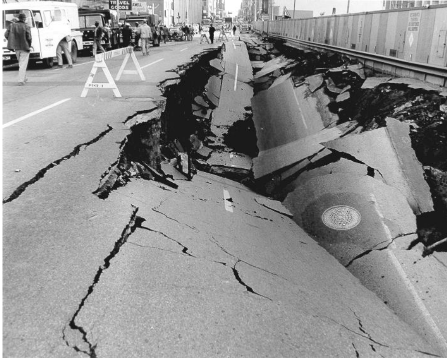
Slide into open excavation and destruction of a section of Elm Street in Dallas. Slide resulted from insufficient fracture investigation in Austin Chalk prior to excavation.
