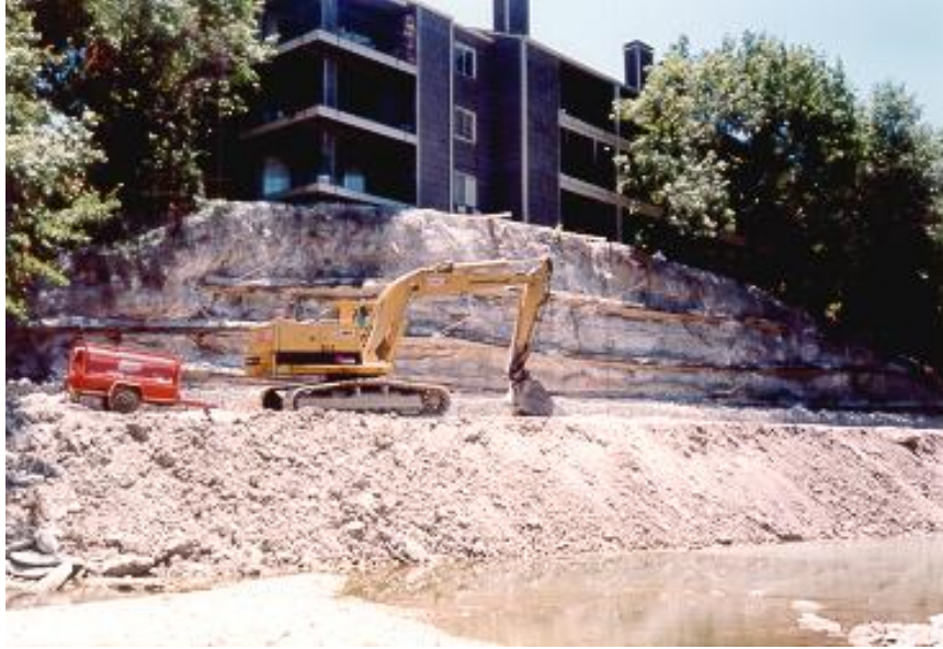
Erosion and steepening of cut bank within Austin Chalk Formation in Dallas area. Note the corner of the apartment foundation has been undermined by the erosion.
