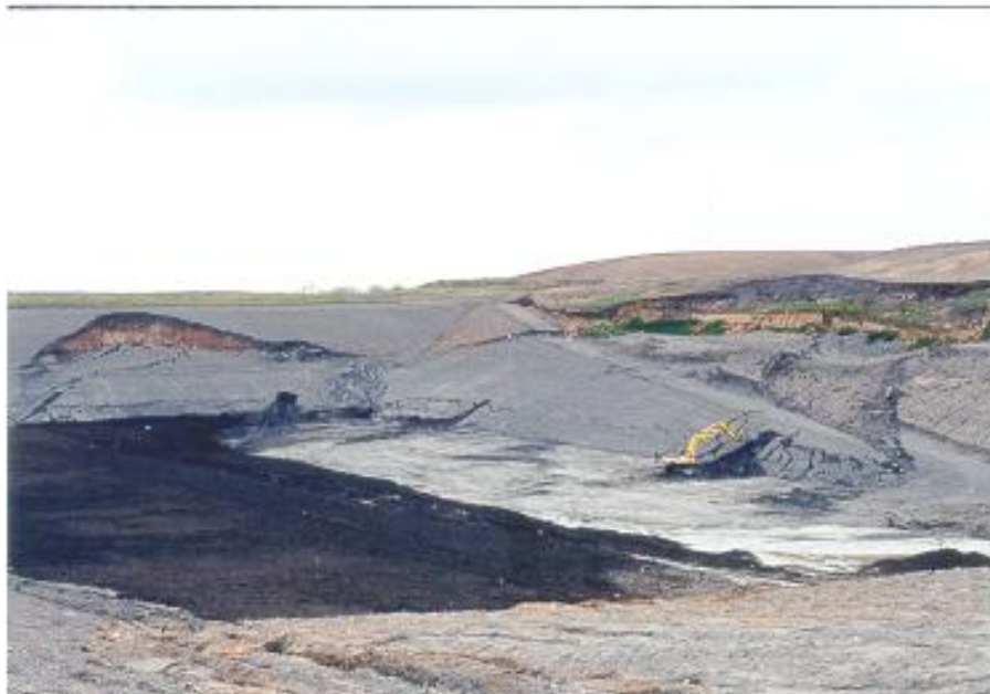
Landslide in high walls of new landfill cell in north Texas resulting from pre-existing geologic conditions.
