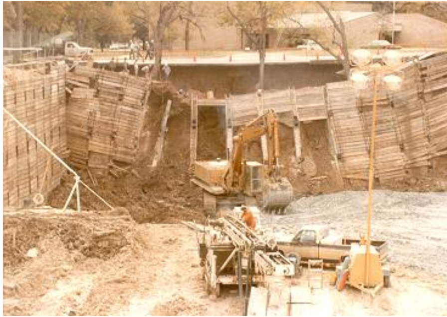
Slide into open excavation on Maple, November 11, 1984. Failure of soldier piles due to inadequate anchoring of piles resulting from lack of investigation of geologic conditions along that section.
