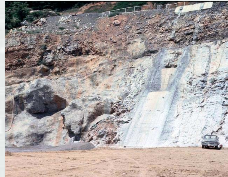
Concrete membrane exposed along the slope of the left abutment, note shotcreting to the left of the membrane
