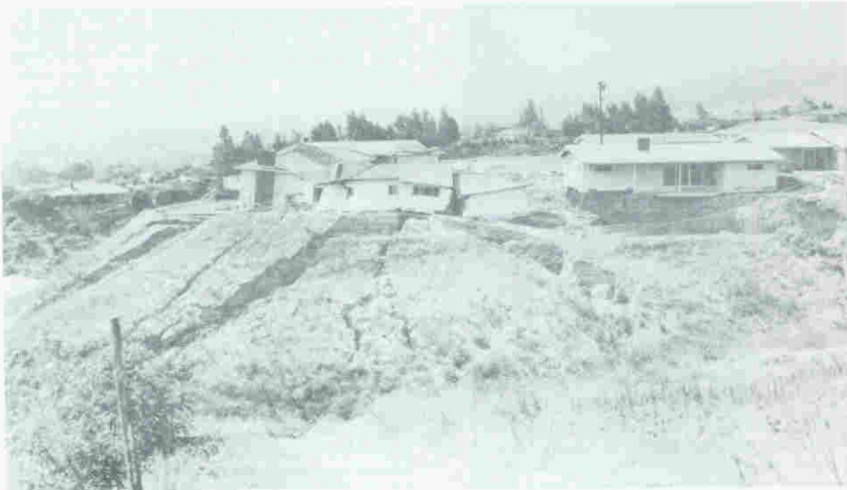
Figure 11. A small slide that destroyed two homes and left a third with only partial support, Rolling Hills Estates in the Palos Verdes Hills. This slippage, which occurred in 1960, was caused mainly by the placing of structures and masses of fill upon an unstable slope.
