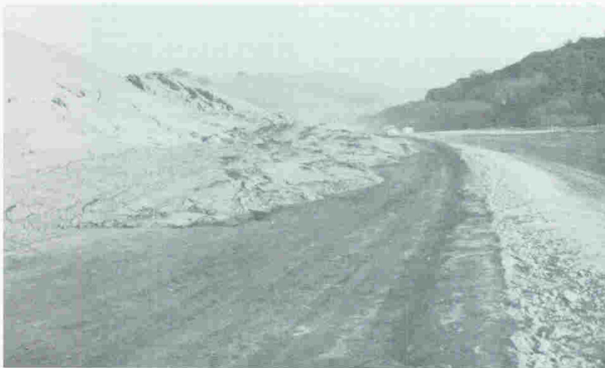
Figure 8. Toe of a landslide that moved across the roadway during construction of Interstate 280 west of Los Altos Hills in November, 1967.
