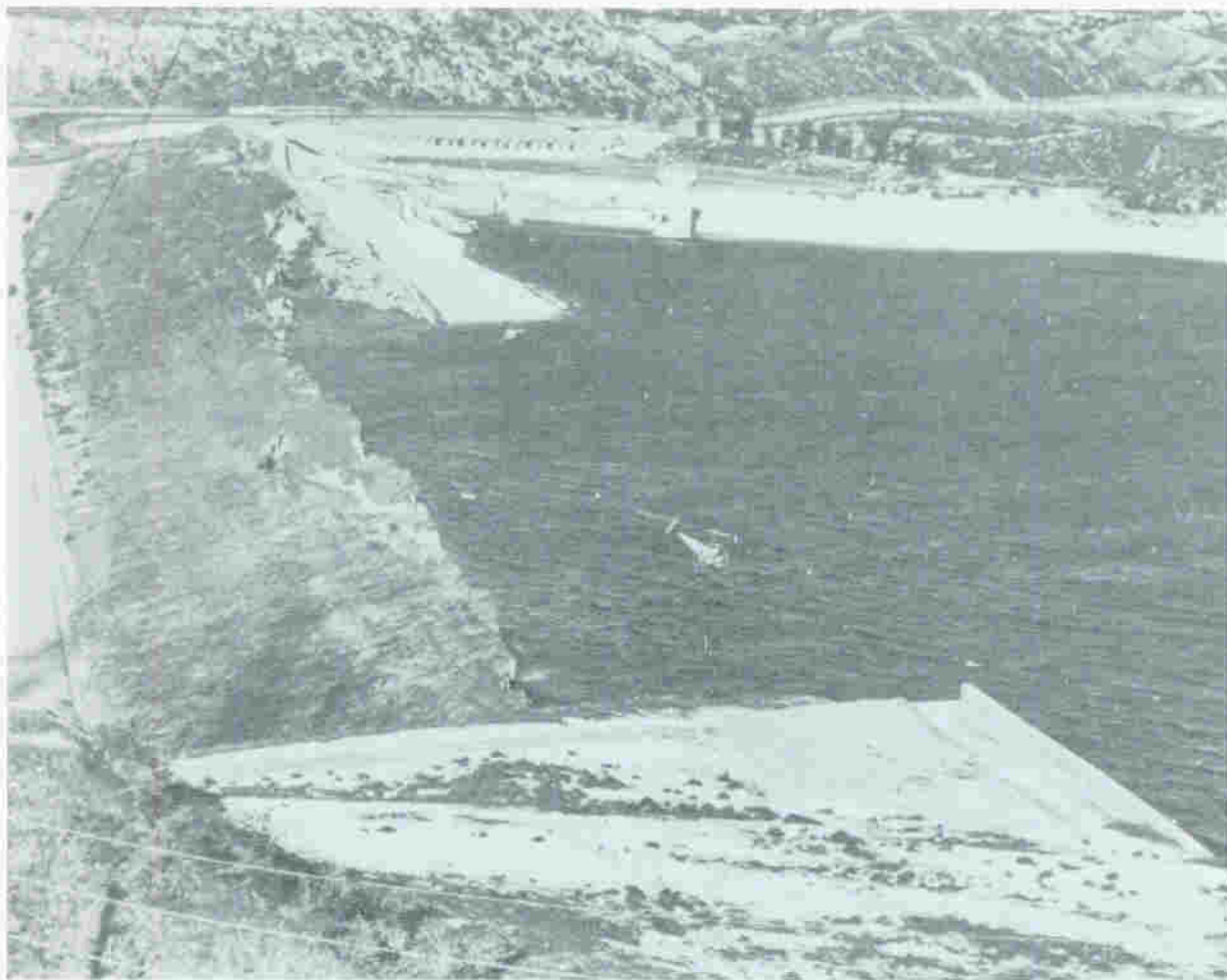
Figure 6. The Lower Van Norman Dam after partial collapse from strong seismic shaking on February 9, 1971. A large portion of the structure has been displaced downward into the reservoir area. Photograph courtesy of Gordon B. Oakeshott, California Division of Mines and Geology.
