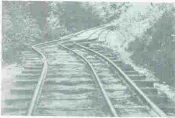
Figure 13. Severe deformation of railroad track during the San Francisco earthquake of 1906, South Pacific Coast Railroad near Wright's Station in the Santa Cruz Mountains. This section of dual-gauge line was kinked and shortened by strong ground motion associated with activity along the nearby San Andreas fault. Photograph from Collection of Roy D. Graves, San Francisco.
