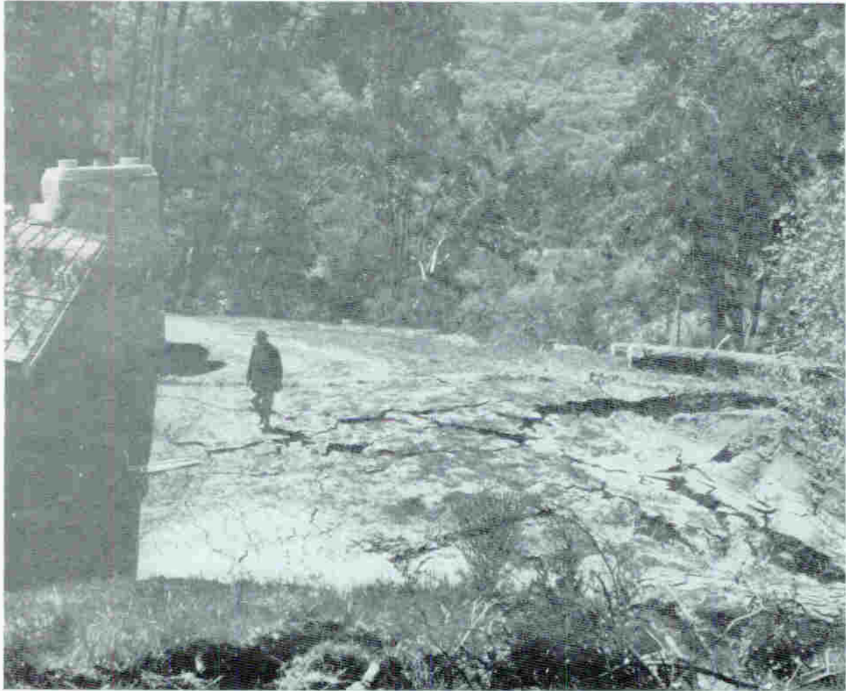
Figure 10. Deep cracks in active landslide mass, Vista Verde area near Portola Valley. The ground movement, which wracked the newly-built home at left, represented 1967 reactivation of part of a large landslide complex that was originally developed in 1890.
